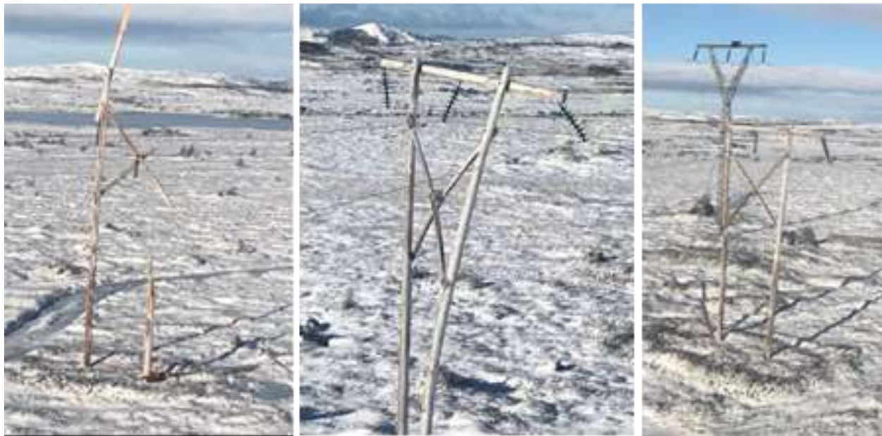
Figure 6: TL219 Structure Failures and Mechanical Bending
