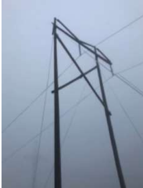
Figure 9: Broken Crossarm on TL203 – Structure 77
