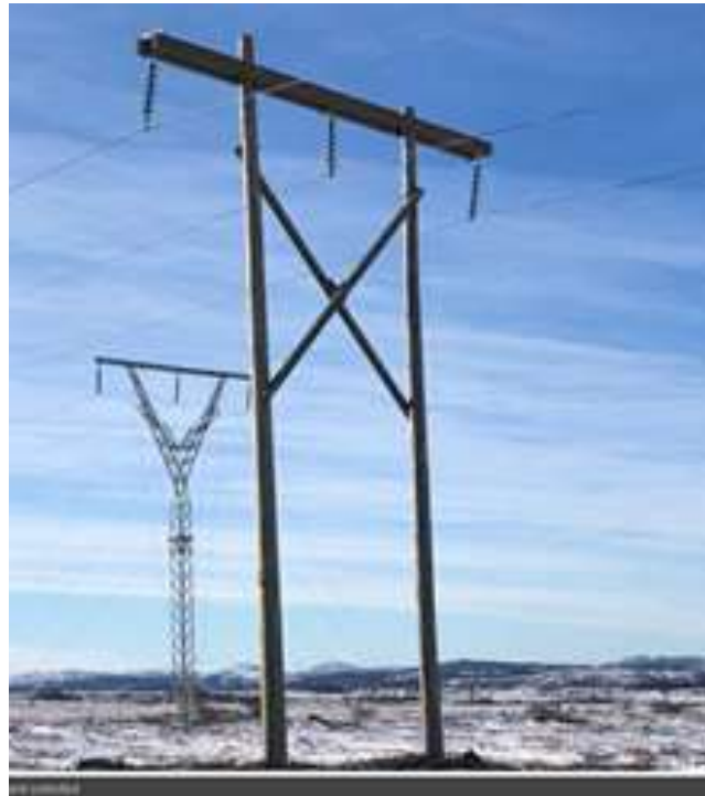
Figure 12: New Tangent Structure (Note TL212 in the Background)
