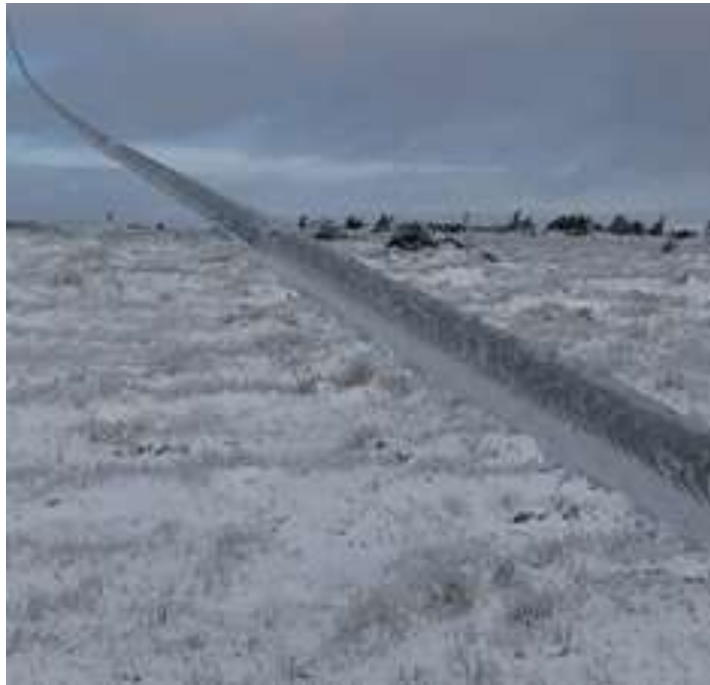
Figure 2: Ice Accumulation on TL219 Conductor
